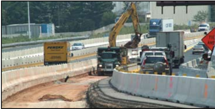
Limited work space is evident on the eastbound Valley Forge on ramp, where stone/asphalt lifts totaling 26" were needed for the new roadway. This section is finished and the construction has moved to the area behind the barrier.
