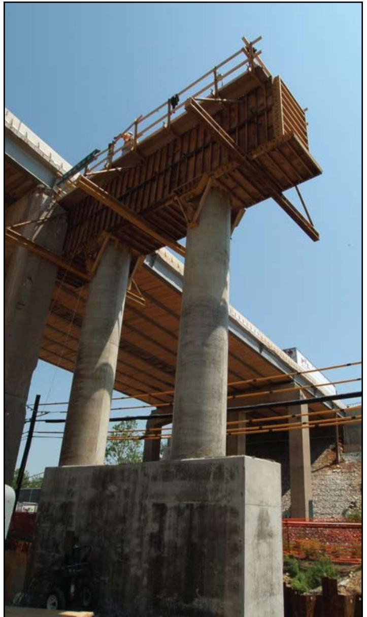
Widening the roadway from four to six traffic lanes required that new reinforced concrete piers for the bridges be constructed adjacent to the existing roadway, allowing little extra room and requiring extreme safety measures.
