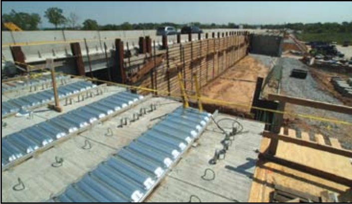
This bridge reconstruction over Henderson Road is one of five required for the Turnpike project. As of this writing, traffic is running over this bridge and the adjacent roadway supported by MSE wall.
