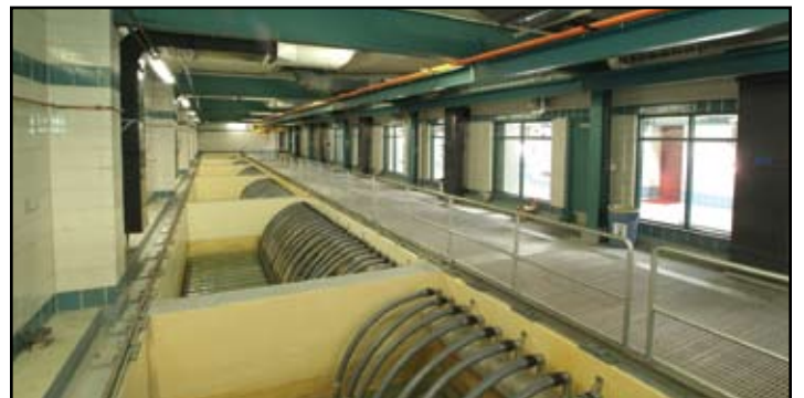
Modified multimedia filters with new membrane filters installed.
