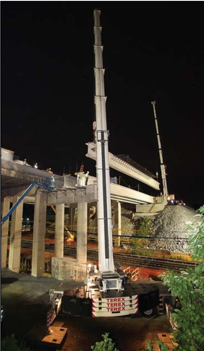
Pre-cast concrete beams are erected over commuter rail line tracks. The center section of the old bridge has now been demolished and new concrete abutment is being placed. Concurrent with this operation is the widening of the opposite side of the roadway.
