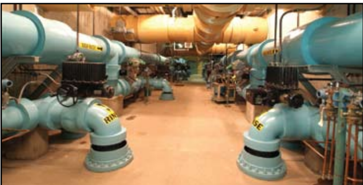
New GAC filter pipe gallery tied into the existing GAC filter pipe gallery.
