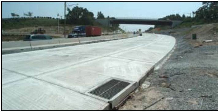
All ramps at the Valley Forge interchange were reconstructed, including the westbound off ramp shown. New embankment has been built and traffic now runs on this side of barrier while the far side is under construction.
